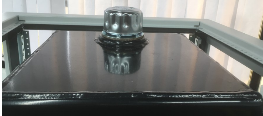
Figure 3: 1 kW Chiller coolant reservoir
